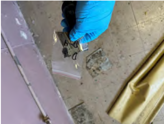
Photo #1 Asbestos floor tile – Basement Room B13. (Sample #D-1)
