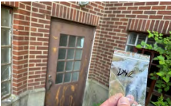
Photo #5 Asbestos containing door caulking (Sample #D42)
