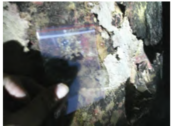
Photo #6 Tank insulation with trace amounts of asbestos– 1 st Floor Room #63 (<1% Chrysotile)
