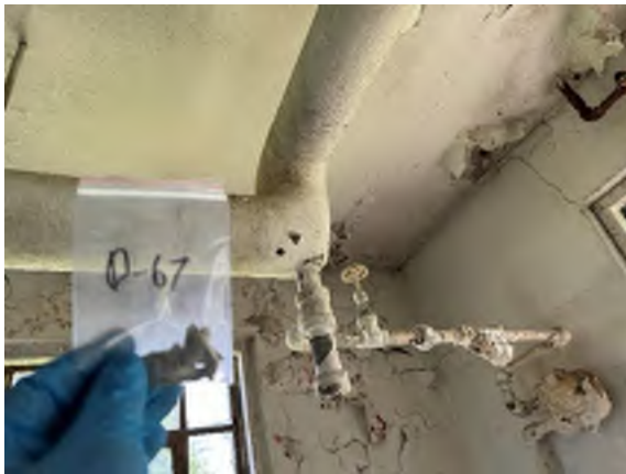
Photo #7 Asbestos containing muddied fitting – Basement Room B5. (Sample #D-67)
