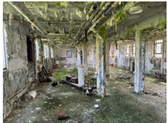
Photo #12 Overview of mold growth and moisture damaged surfaces on basement level.
