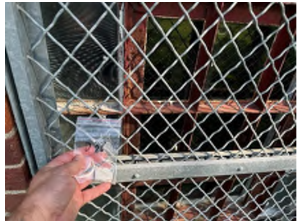
Photo #4 Asbestos containing window glazing (Sample #D38)).
