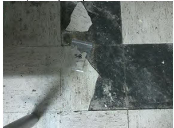
Photo #4 Asbestos containing floor tile (Tan) – 2 nd Floor Room #31 (2% Chrysotile).
