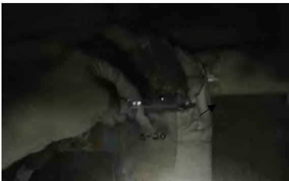
Photo #5 Asbestos containing mudded pipe fitting – 1 st Floor Room #63 (10% Chrysotile)
