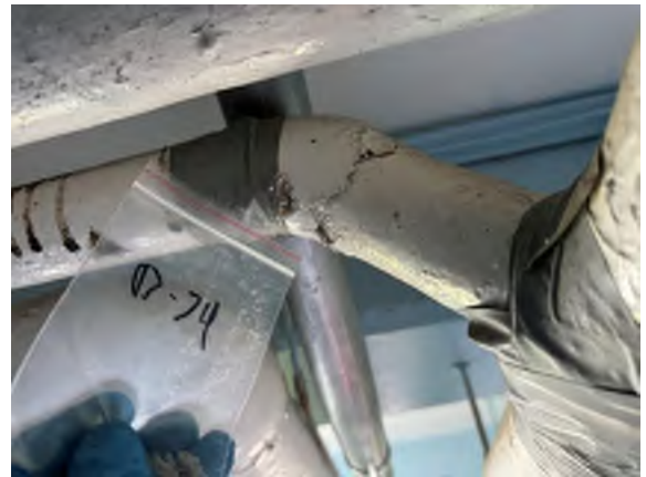
Photo #8 Asbestos containing muddied fitting – Basement Room B14. (Sample #D74)
