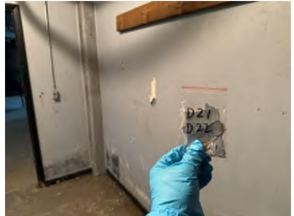
Photo #2 Asbestos containing drywall mud – Basement Room B16. (Sample #D22)
