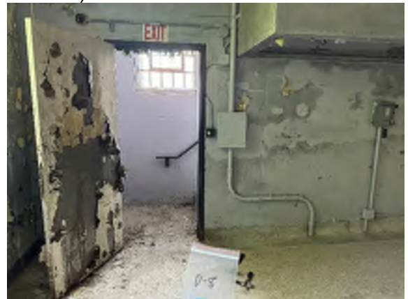
Photo #10 Overview of peeling paint on basement level surfaces.
