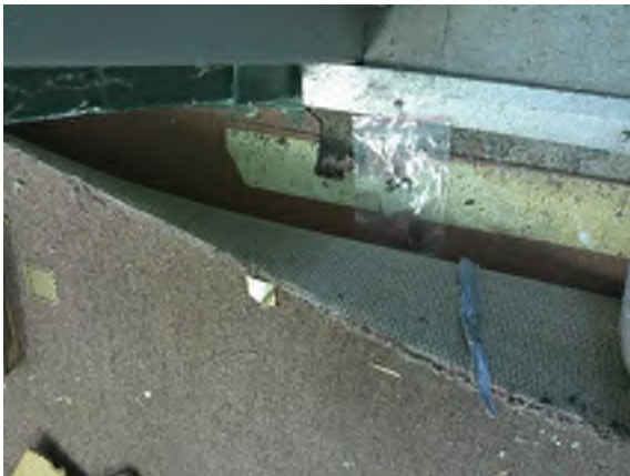
Photo #3 Asbestos containing floor tile (Red w/ Pits) – 2 nd Floor Room #2 (2% Chrysotile)
