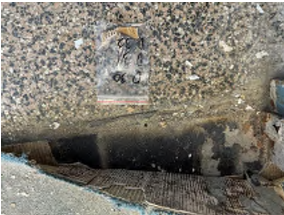
Photo #3 Asbestos containing floor tile mastic 1 st Floor Room #126 (Sample #D32))
