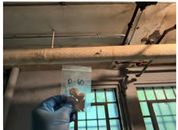
Photo #6 Asbestos straight pipe insulation - Basement Room #B16 Sample #D60)
