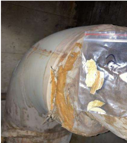
Photo #1 Asbestos: Sample #2. White Pipe End Caulk/Sealant. Same material observed on Pipes G & F throughout.
