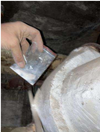
Photo #3 Asbestos: Sample #4 – 10"-12" O.D Valve Insulation White Section #1 Pipe H.
