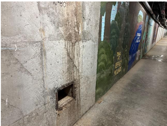
Photo #5 Inside the E 13 th Street tunnel, looking at one of the vents.
