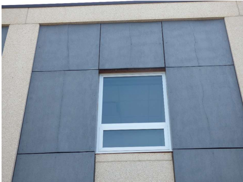
Cracked boards found on the facade
