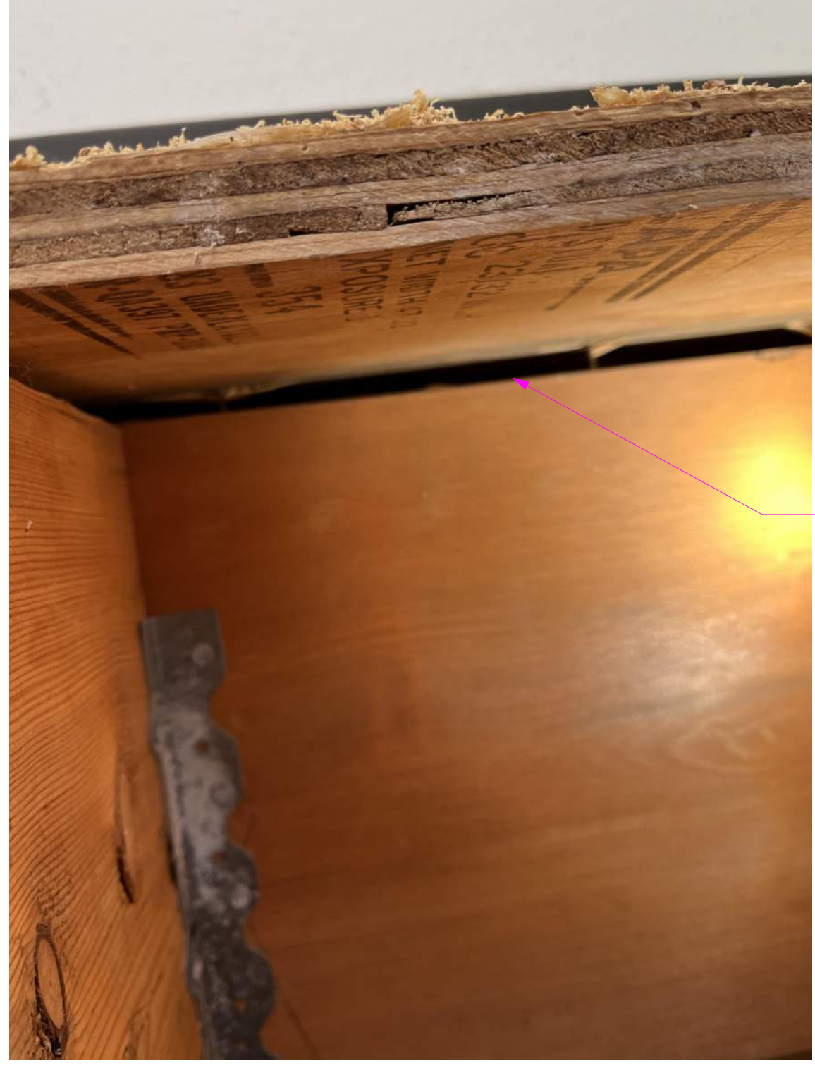
APPROXIMATE 3/4" GAP BETWEEN JOIST AND PLYWOOD SUBFLOOR
