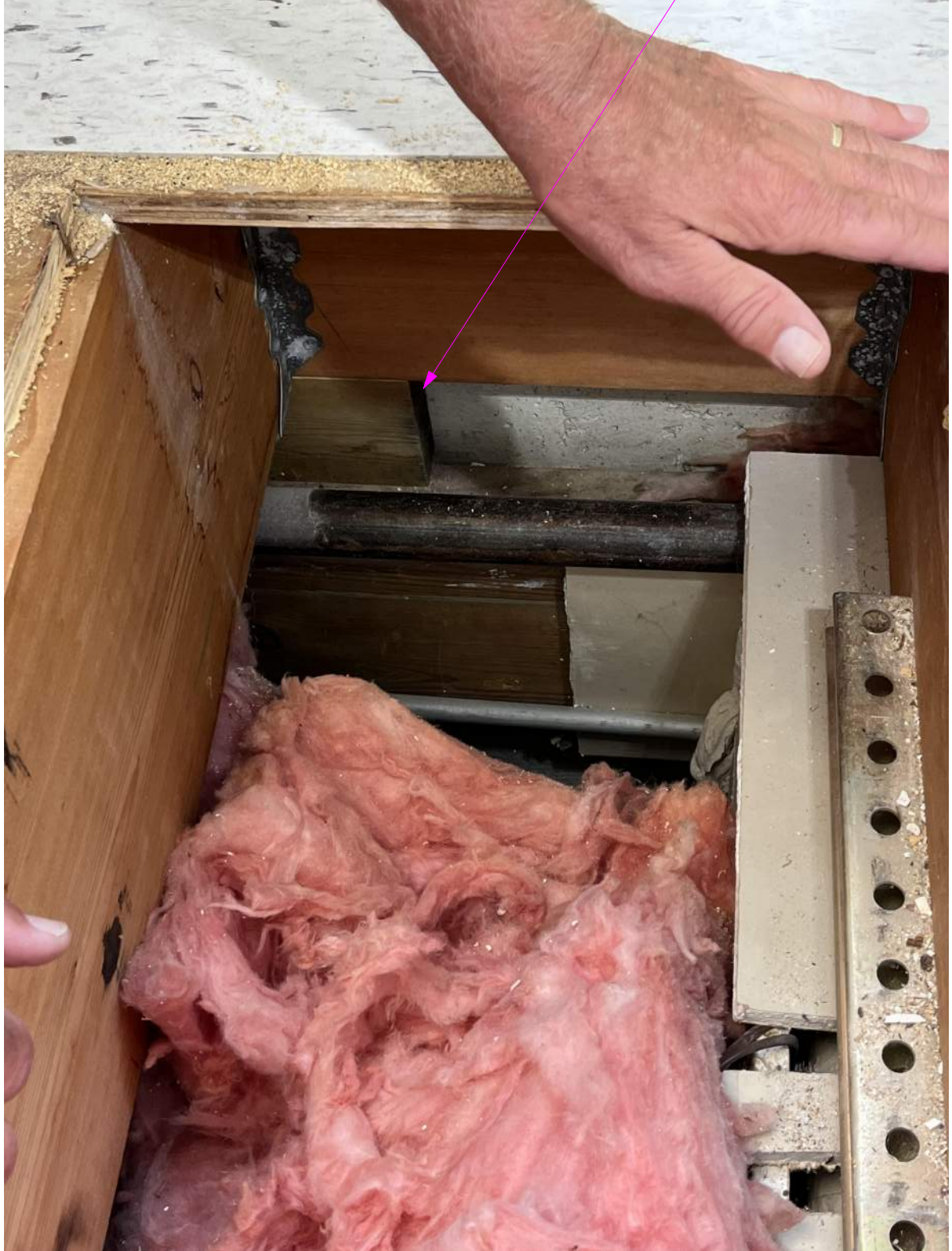
HEADER IS RESTING ON 2X4 POST, INTERMITTENTLY
