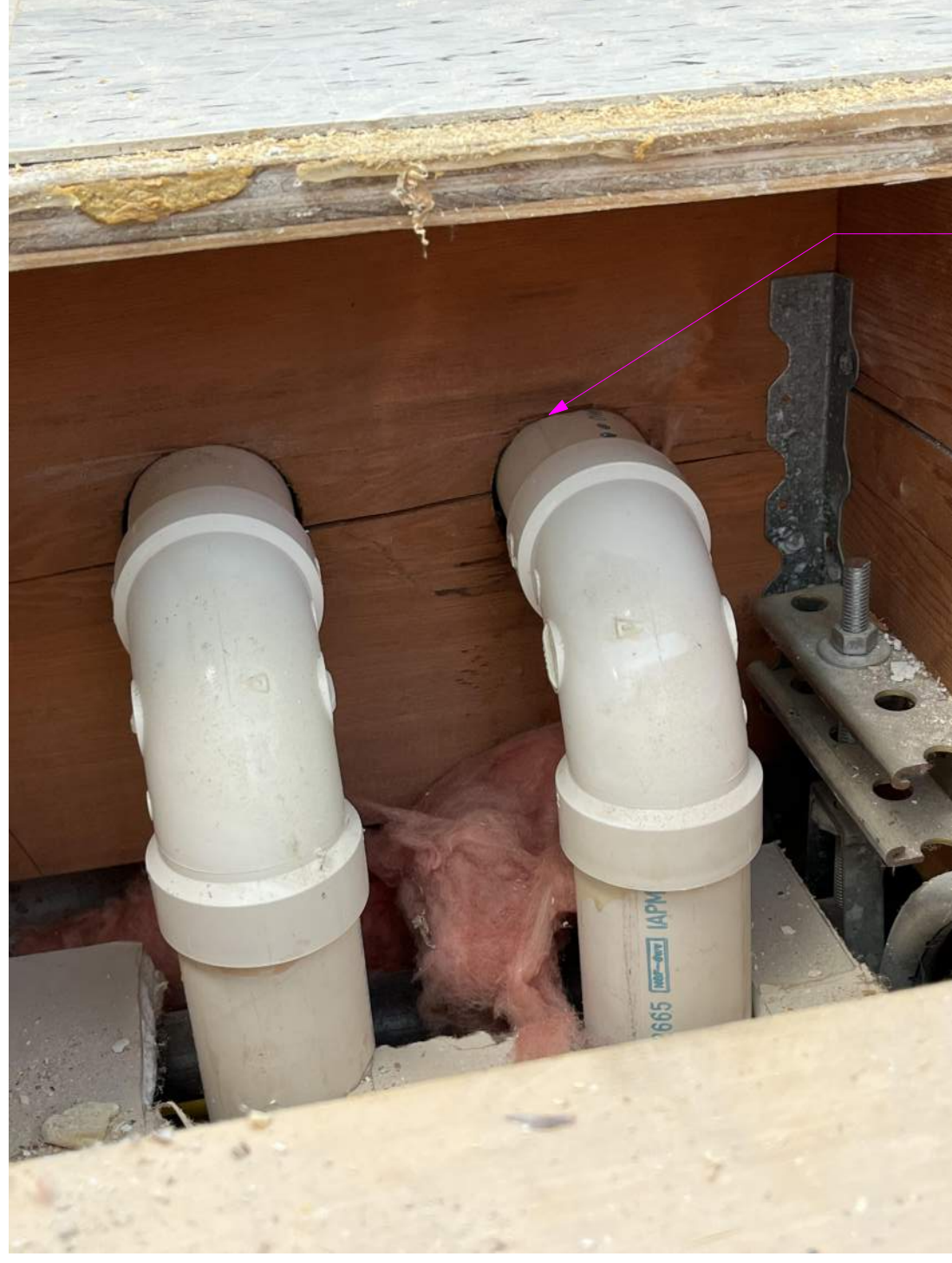
HEADER IS BEARING ON PVC PIPES
