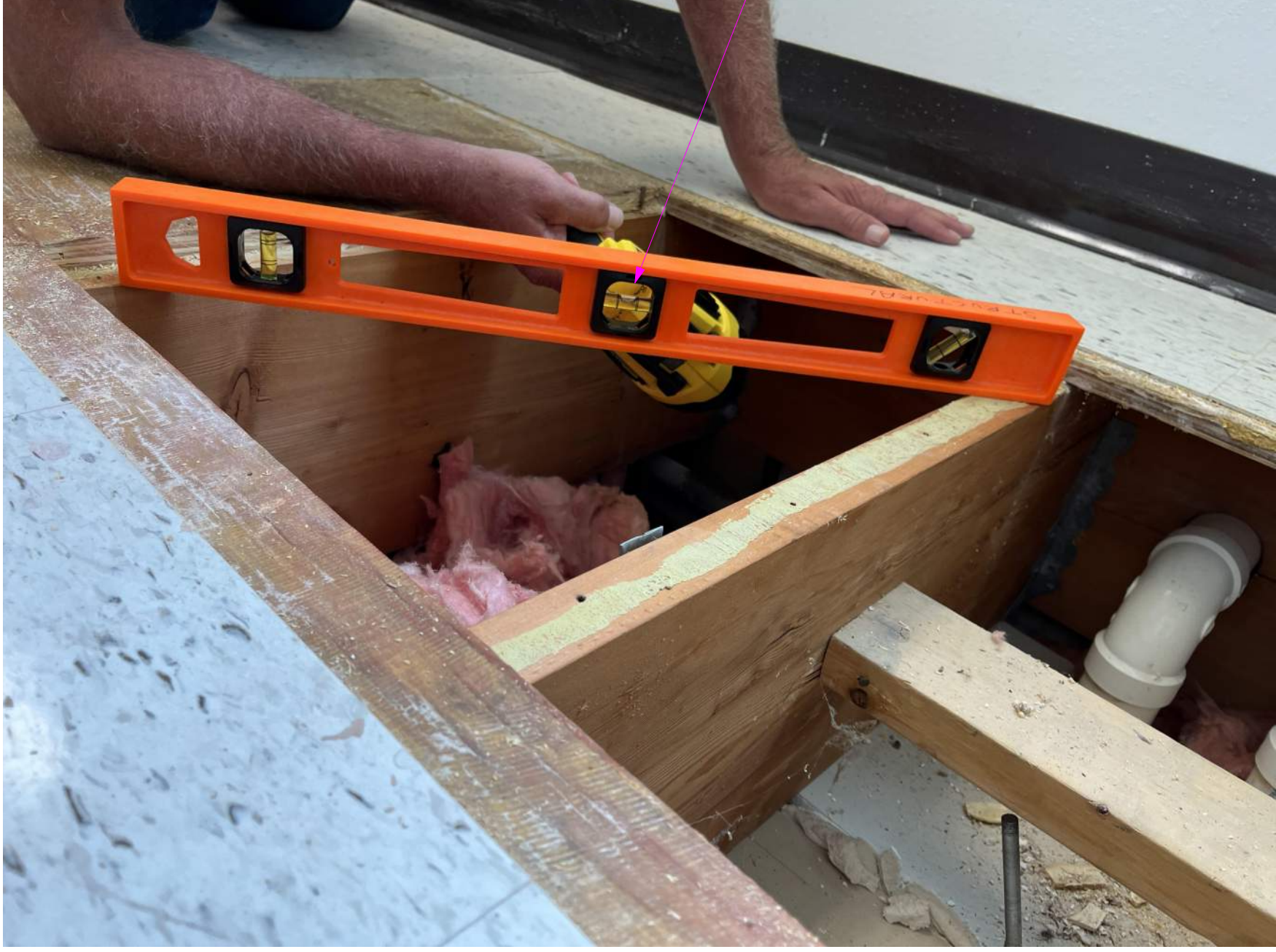
JOISTS ARE LEVEL WITH EACH OTHER AFTER DROPPING 3/4" FROM THE SUBFLOOR
