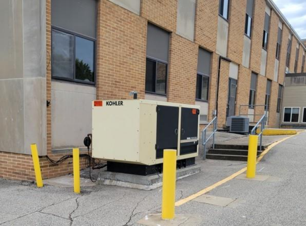
Sac City HS Generator
