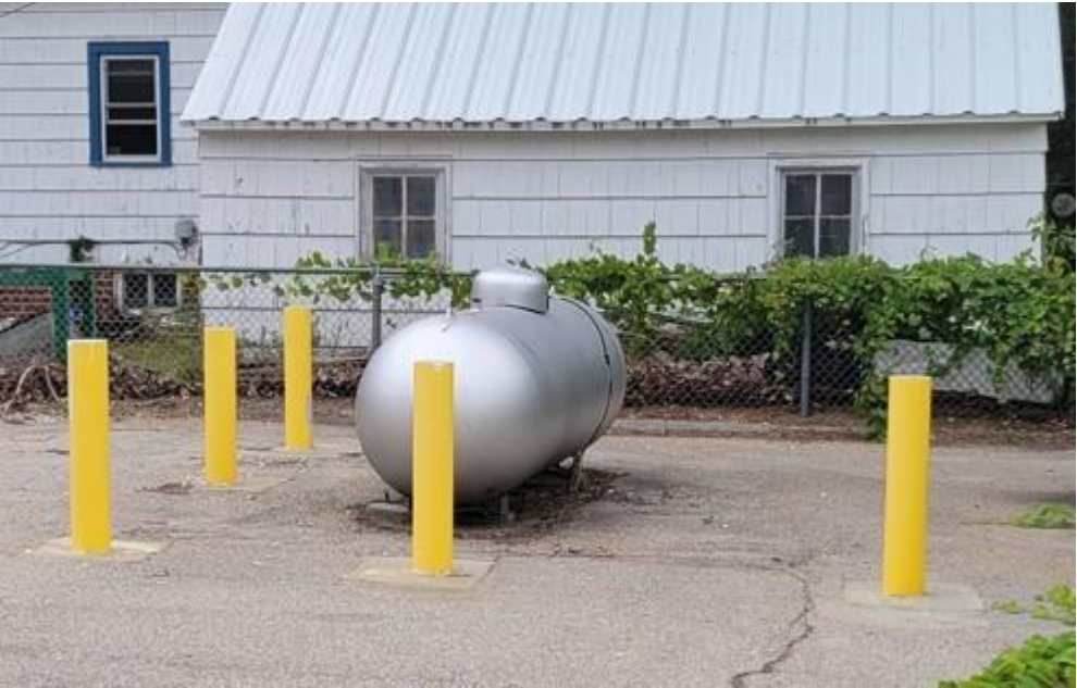
Sac City HS Propane Tank
