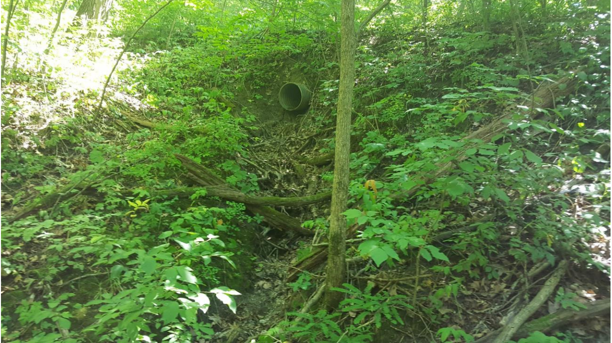
This culvert, the second area of concern, is at the north end of the roadway section in question; it is approximately 8-feet from the edge of the roadway.
