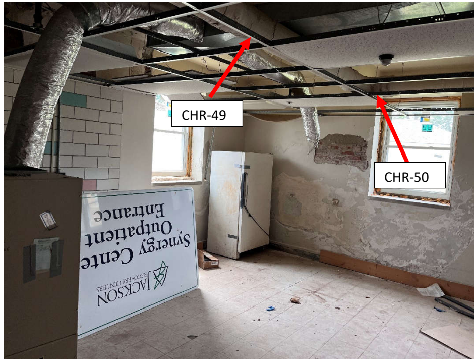
View of Asbestos containing TSI Hardpack Run and TSI Hardpack Elbow (Samples CHR-49, 15% Chrysotile and CHR-50, 5%-20% Chrysotile)
