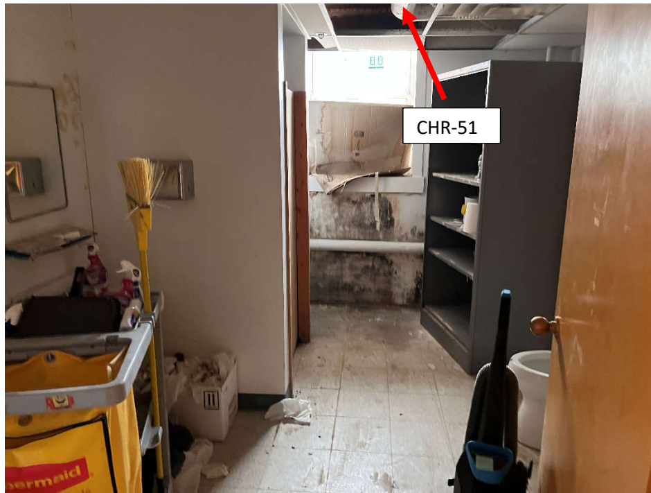
View of Asbestos containing Aerocell (Samples CHR-51, 20%-35% Chrysotile)
