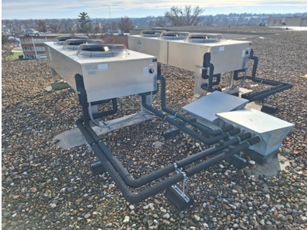
DACK ROOF - COOLING UNIT CURBS & PIPES
