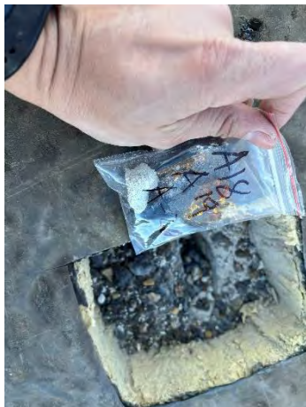
Photo #5 Sample A-12, 18, 27, 34 Black Roof Tar, Malloy Building ( 5-20% Chrysotile )
