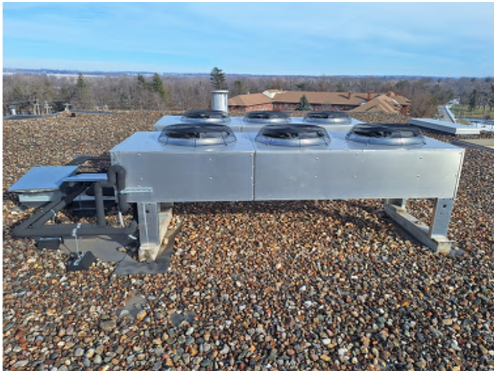
DACK ROOF - COOLING UNITS
