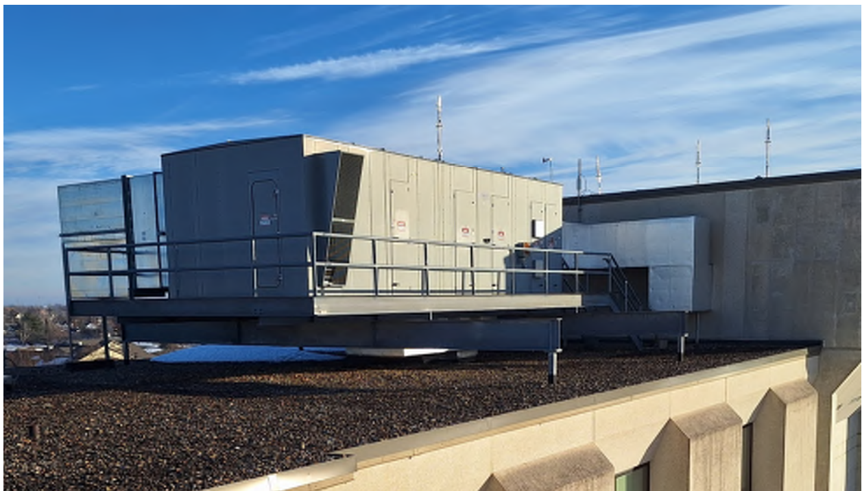
MALLOY ROOF - RTU & SUPPORT BEAMS ON WEST SIDE
