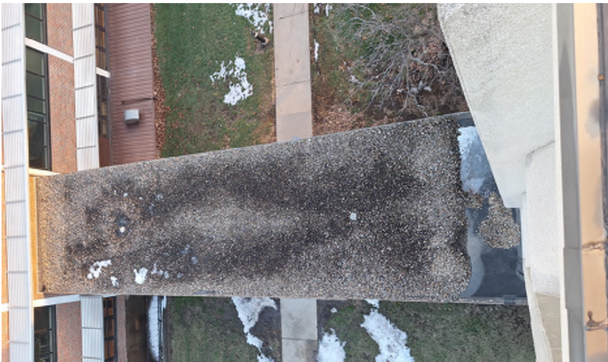
MALLOY -LOFTUS CONNECTING COORIDOR ROOF
