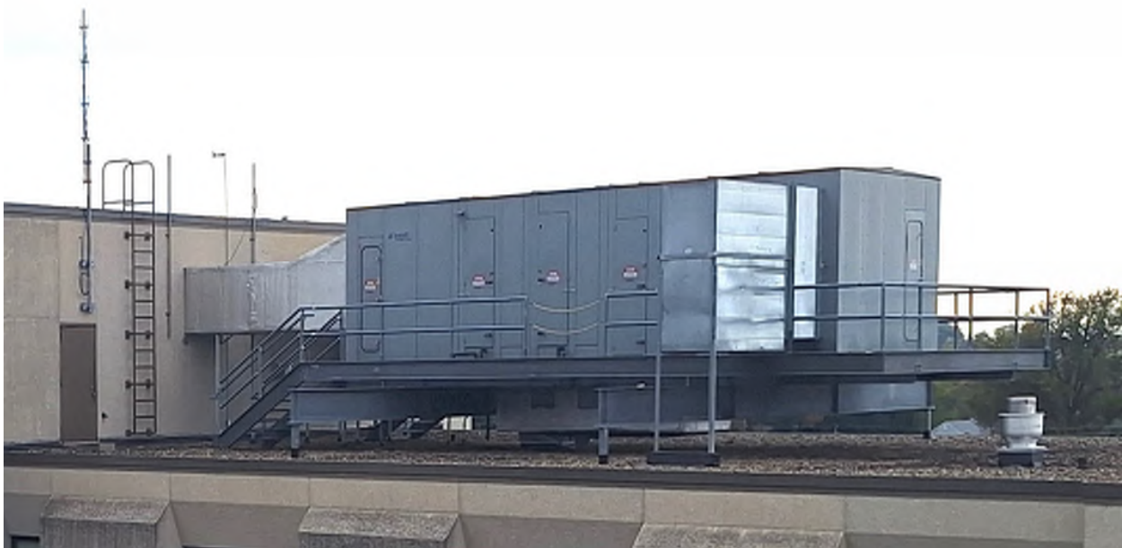
MALLOY ROOF - LARGE RTU
