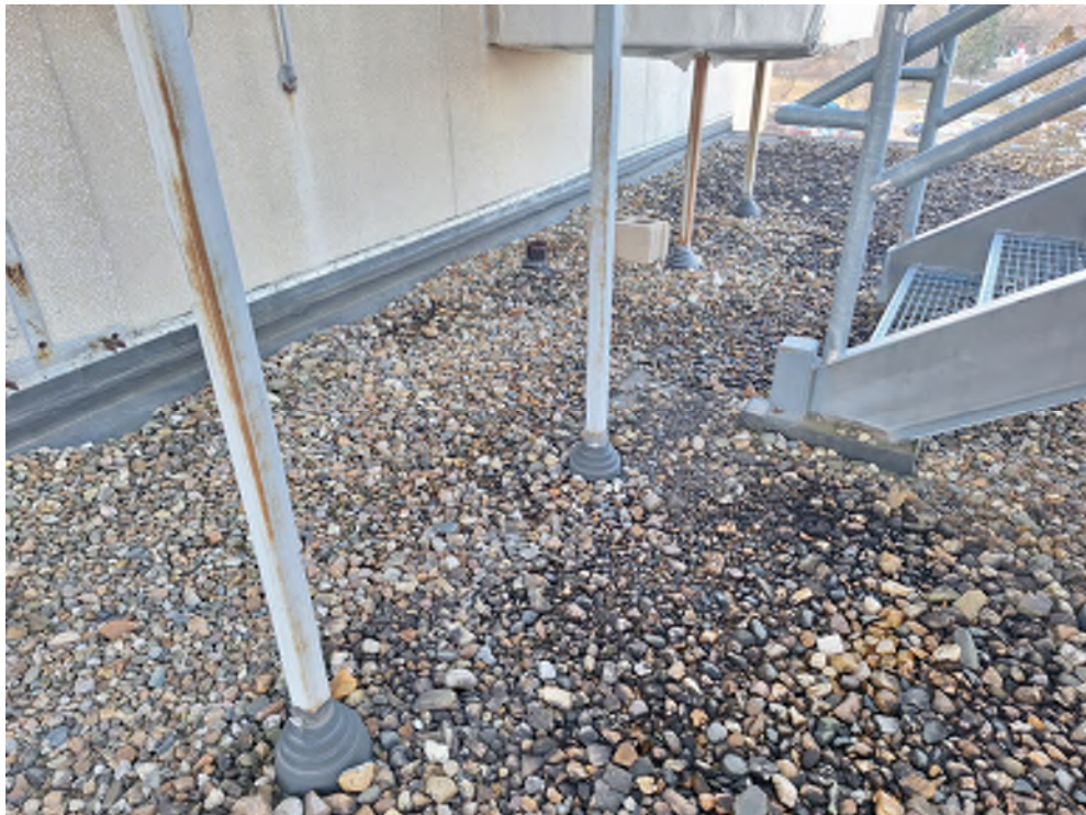
MALLOY ROOF - PIPE SUPPORTS & STAIRS AT RTU
