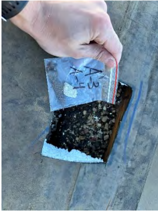
Photo #1 Sample A-24 Black Roof Tar, Dack Building ( 15% Chrysotile )
