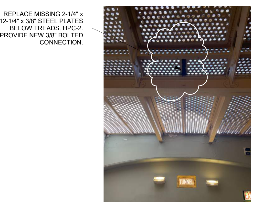
F7 SIDEWALK LIGHT - MISSING STEEL 1" = 1'-0"
