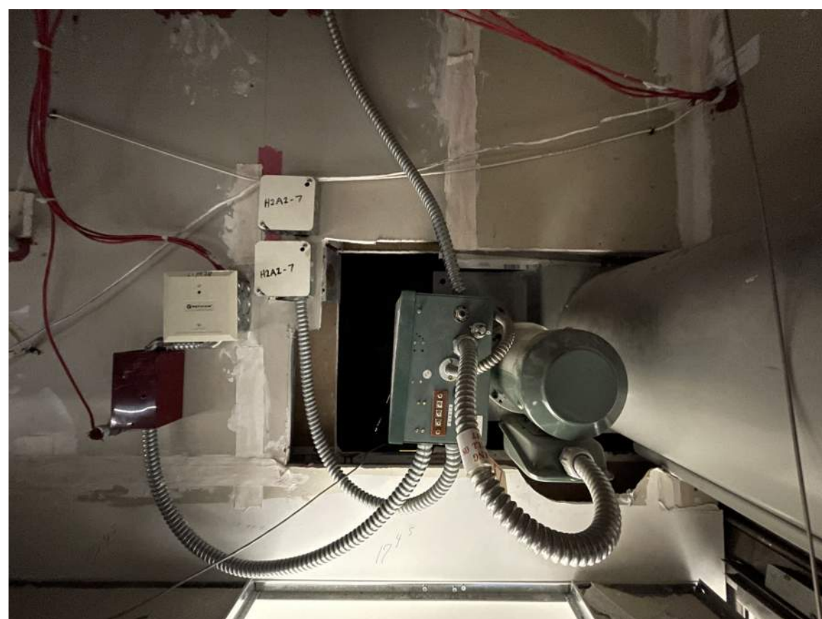
F7 ROLLING DOOR MOTOR LOOKING EAST 1" = 1'-0"
