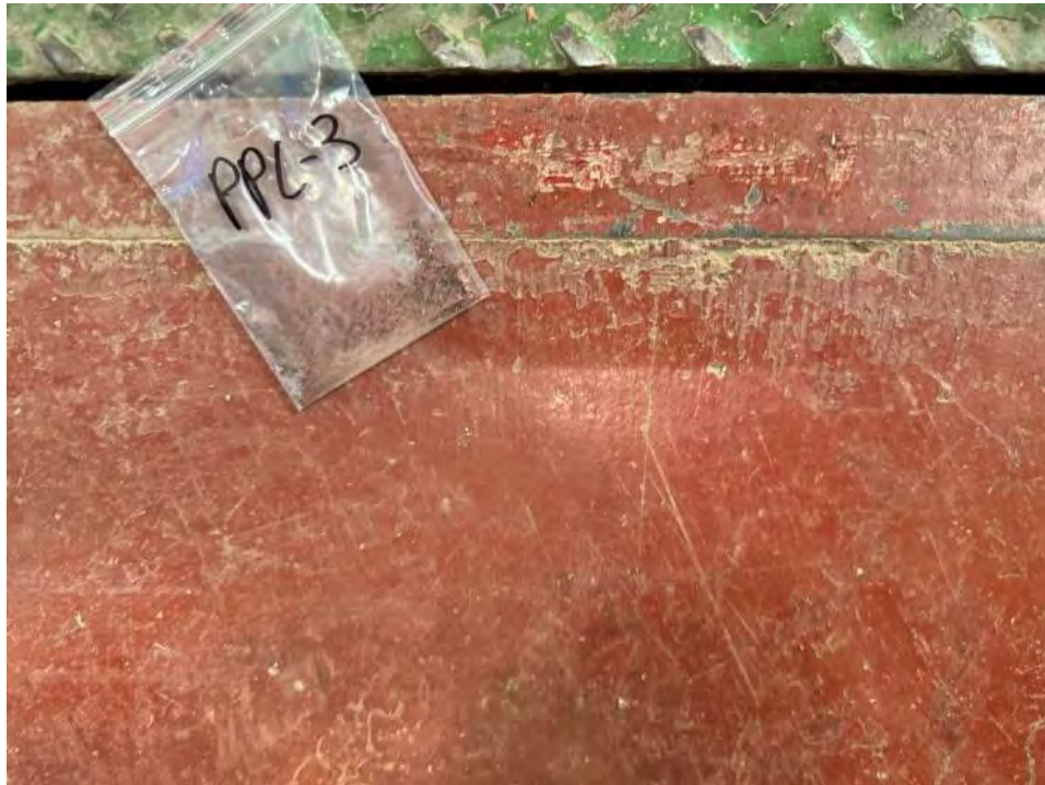
View of the Red Lead Based Paint. (PC-3, 1.0% Pb)
