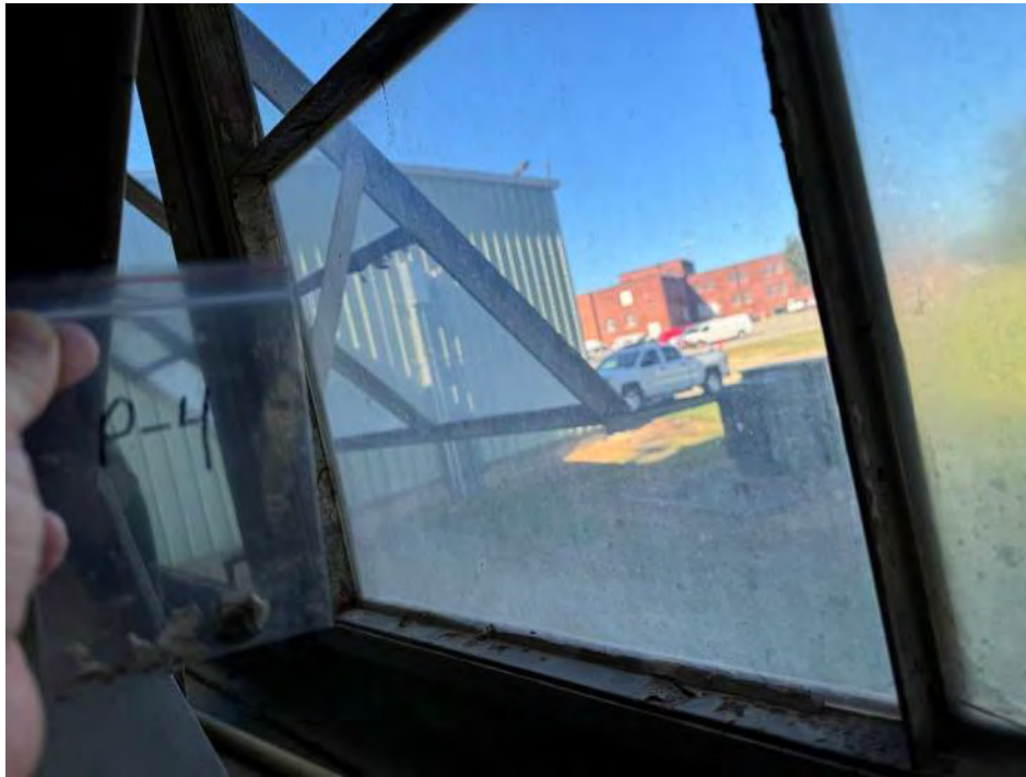
View of the Asbestos Containing Window Glazing. (P-4, 4% Chrysotile)
