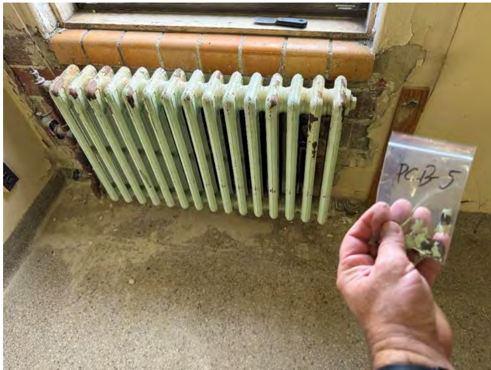
View of the Blue-Green Lead Based Paint. (PCB-5, 0.64% Pb)
