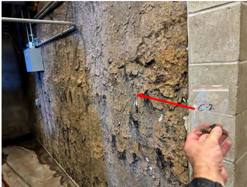
View of the Asbestos Containing Black Tar on dividing wall. (C-2, 8% Chrysotile)
