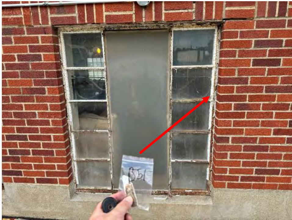
View of the Asbestos Containing Window Glazing. (B-51, 5% Chrysotile)
