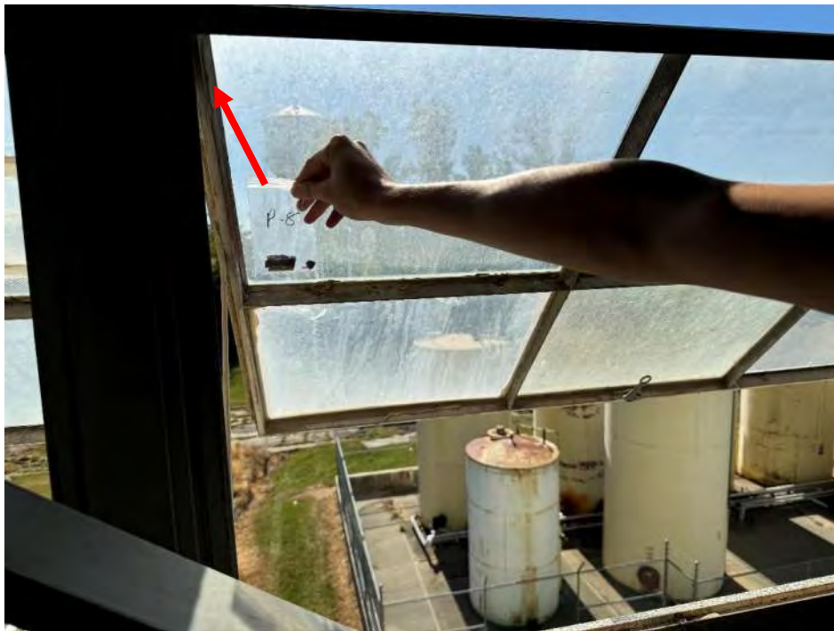
View of the Asbestos Containing Window Glazing. (P-8, 5% Chrysotile)
