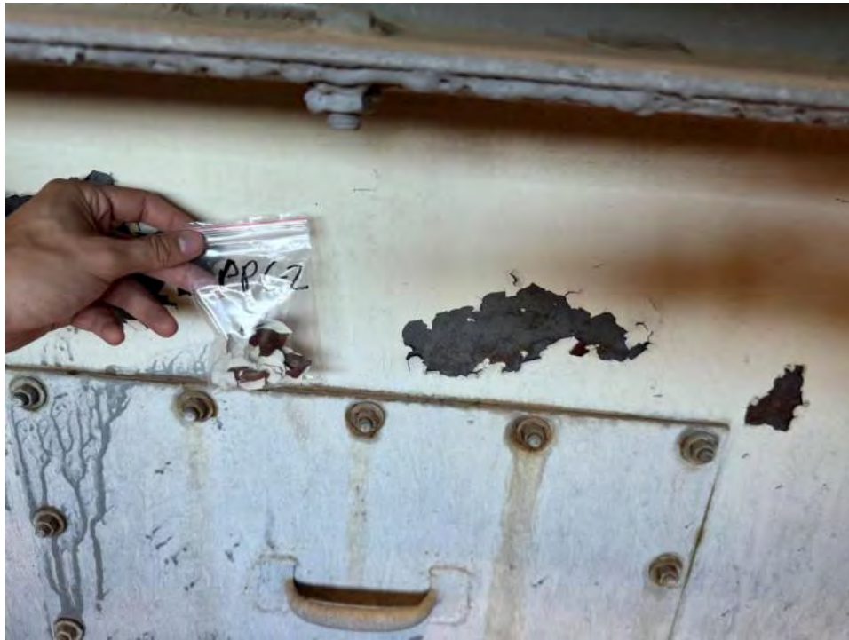
View of the Off-White Lead Containing Paint. (PC-2, 0.32% Pb)
