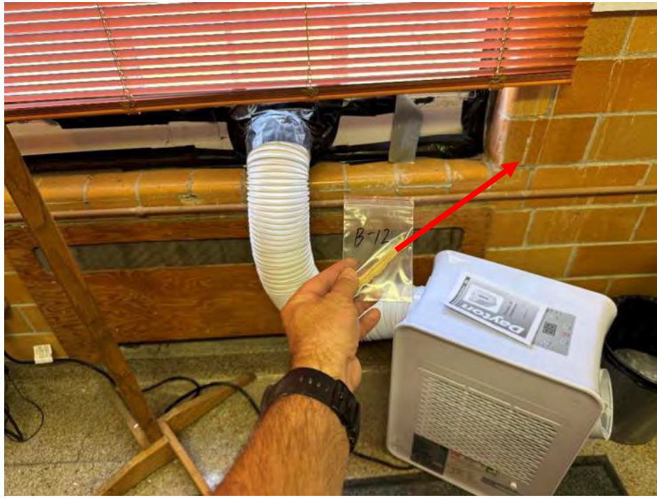
View of the Asbestos Containing White Caulk. (B-12, 6% Chrysotile)
