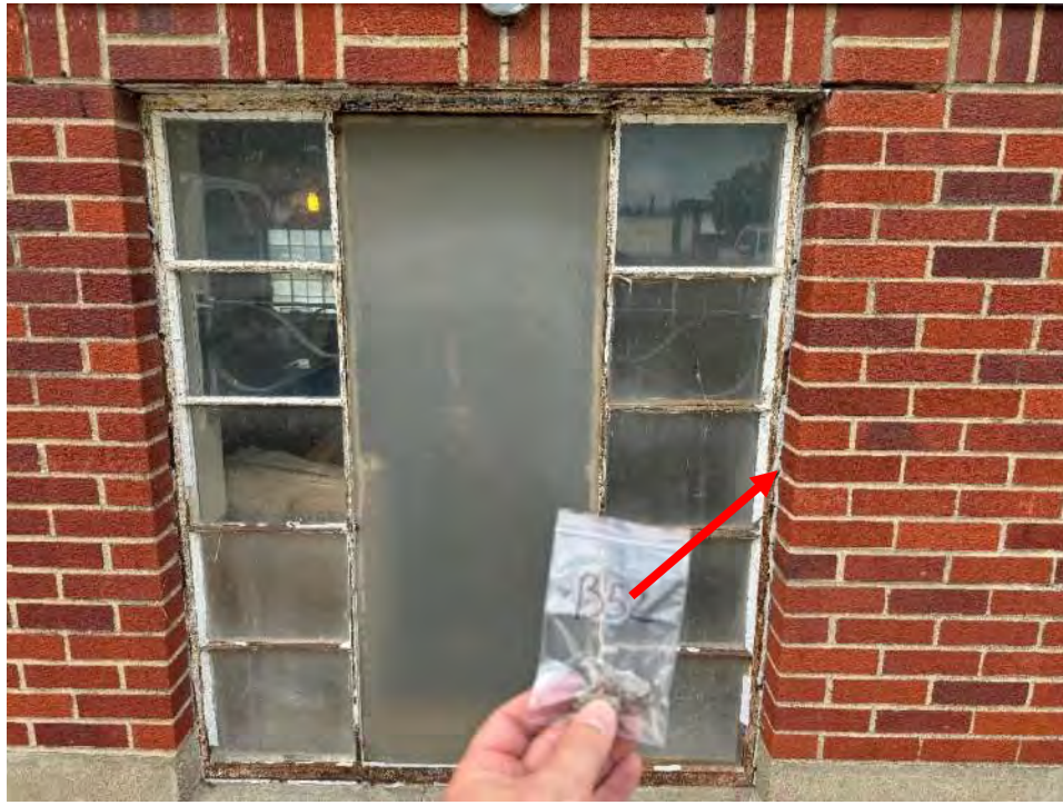
View of the Asbestos Containing Gray Window Caulk. (B-52, 10% Chrysotile)
