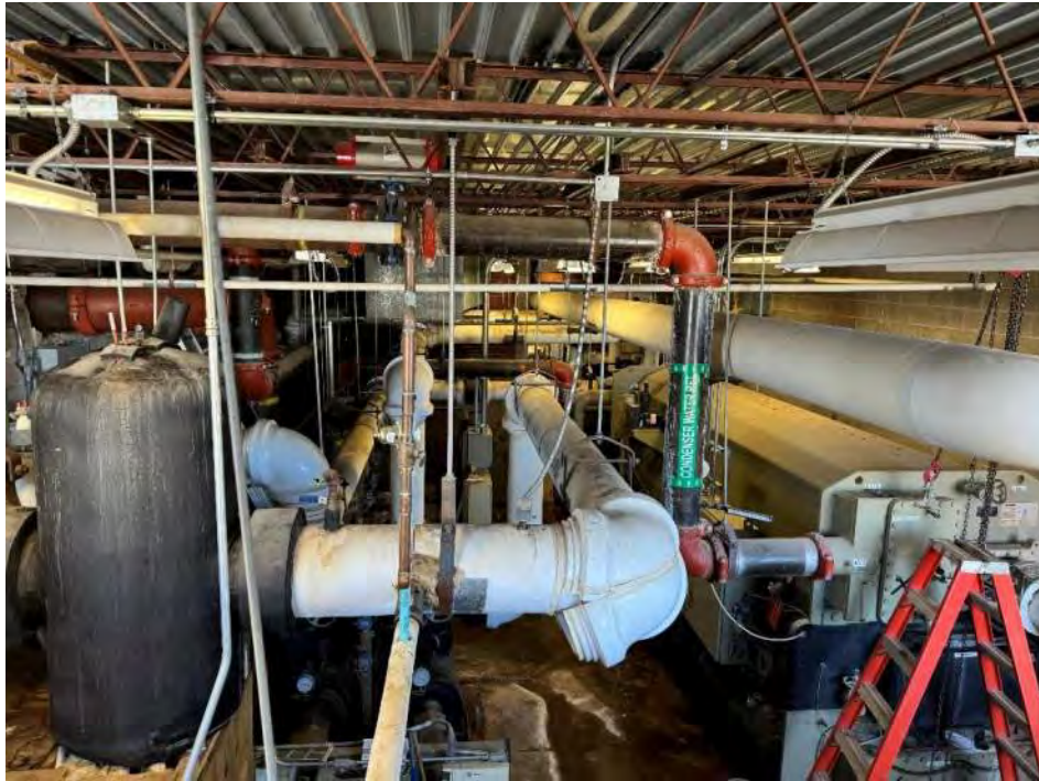
View of the interior of the Chiller Building
