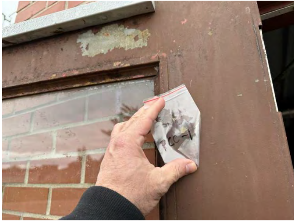
View of the Rust/Brown Lead Containing Paint. (PCC-1, 0.039% Pb)
