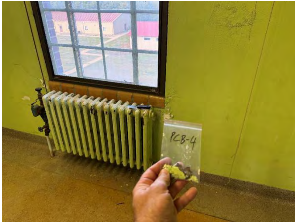
View of the Green Lead Containing Paint. (PCB-4, 0.46% Pb)
