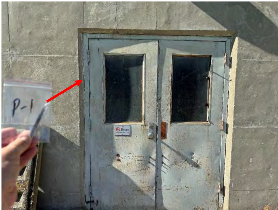
View of the Asbestos Containing White, Brittle Caulk. (P-1, 5% Chrysotile)
