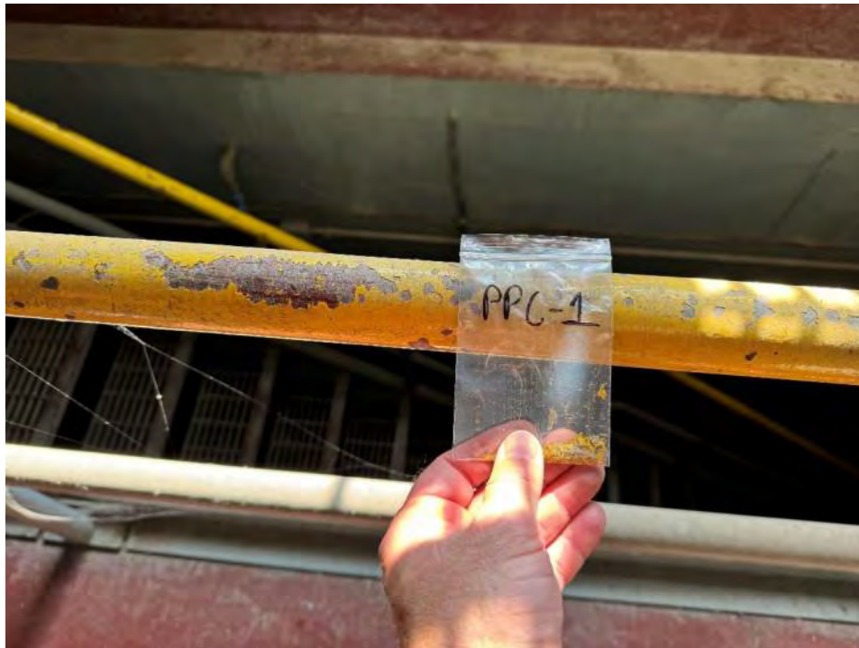
View of the Yellow Lead Based Paint. (PC-1, 20% Pb)
