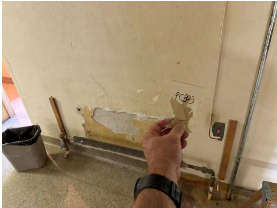
View of the Yellow Lead Containing Paint. (PCB-3, 0.14% Pb)
