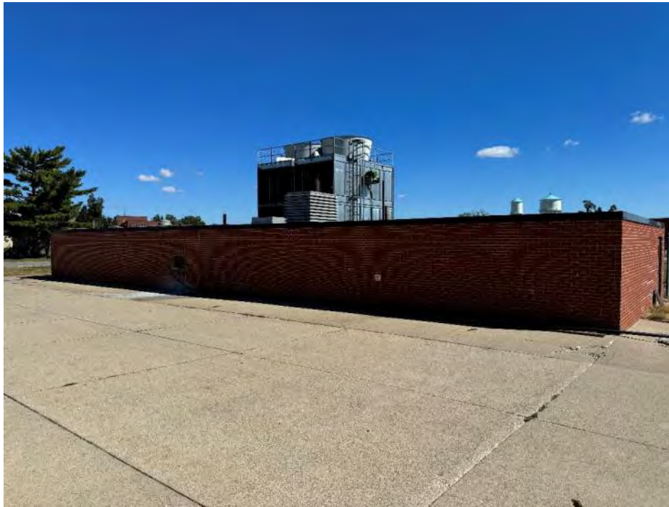
View of the Chiller.
