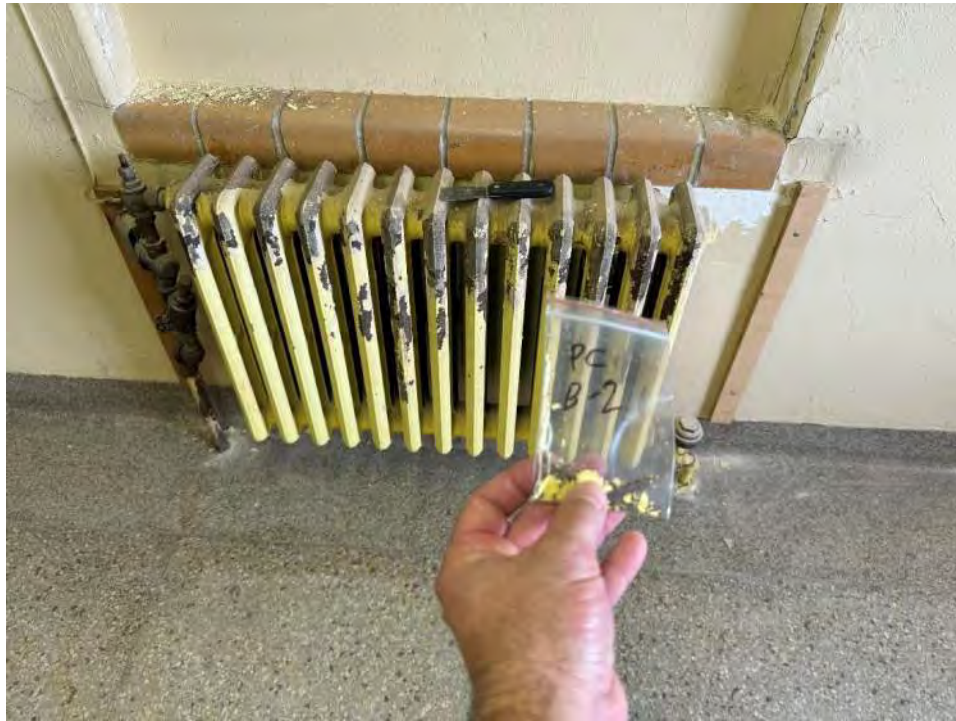
View of the Yellow Lead Containing Paint. (PCB-2, 0.49% Pb)
