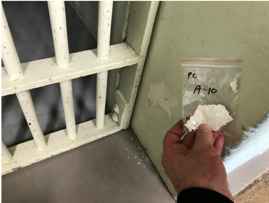
View of the Green Lead Containing Paint on Door Frame (PC A-10, 0.014% Pb).
