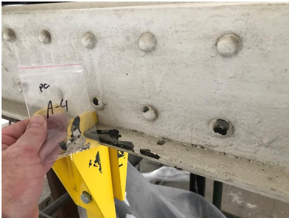
View of the White Lead Containing Paint on Trusses (PC A-4, 0.26% Pb).
