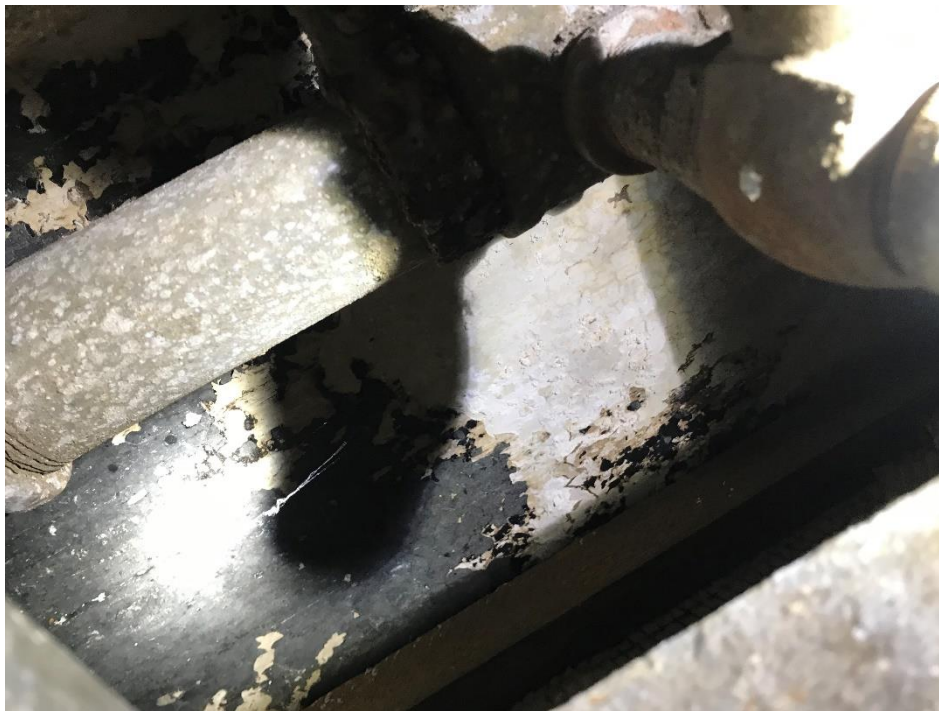
View of the Black Lead Containing Paint inside Pipe Chase (PC A-14, 0.17% Pb).
