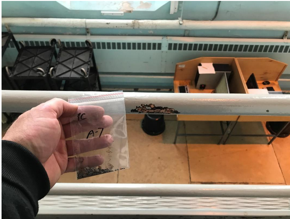
View of the Gray Lead based Paint on Handrails (PC A-7, 5.0% Pb).
