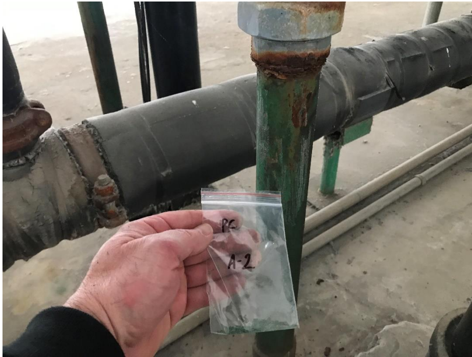
View of the Green Lead Containing Paint on Pipes (PC A-2, 0.34% Pb).
