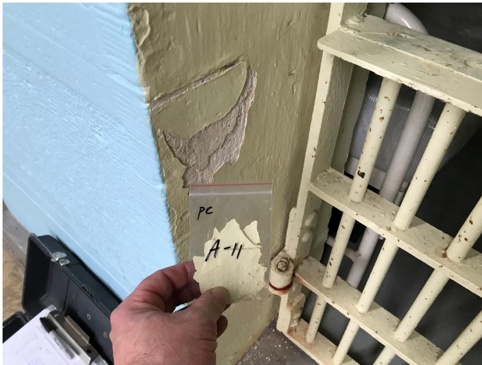
View of the Yellow Lead Containing Paint on Door Frame (PC A-11, 0.048% Pb).
