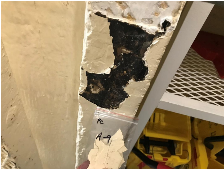
View of the Cream Lead Based Paint on Door Frame and Walls (PC A-9, 2.2% Pb).
