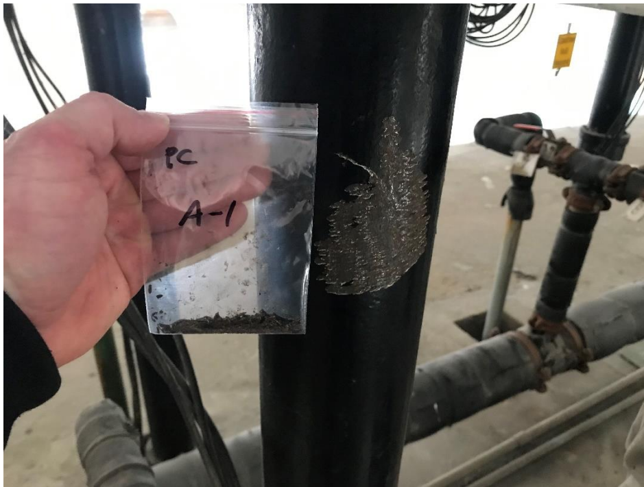
View of the Black Lead Containing Paint on Pipes (PC A-1, 0.017% Pb).
