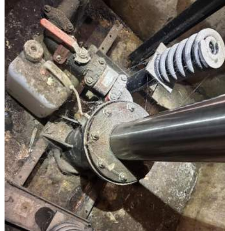
Photo #2 Equipment at Bottom of Elevator Shaft
