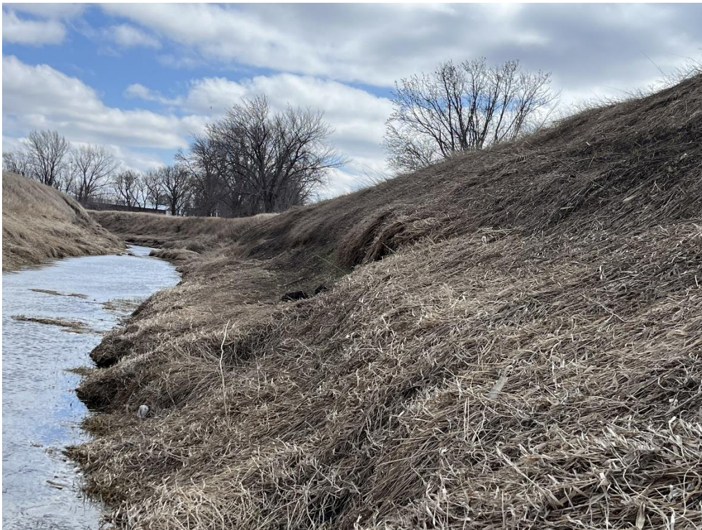
Photo looking south (Moline wetland to right) Previously failed area near Sections 1 and 2 shown
