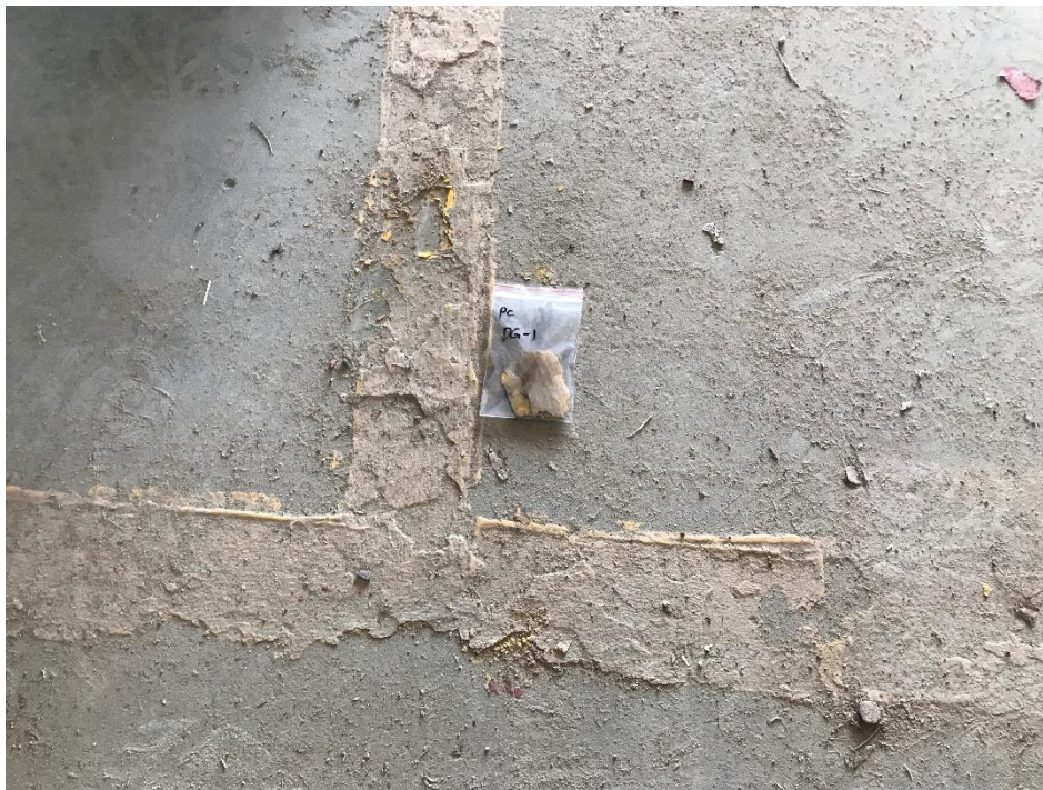
Yellow paint chip sample #1 from floor in the garage (bays 2 & 3) Contains Lead-based paint.
