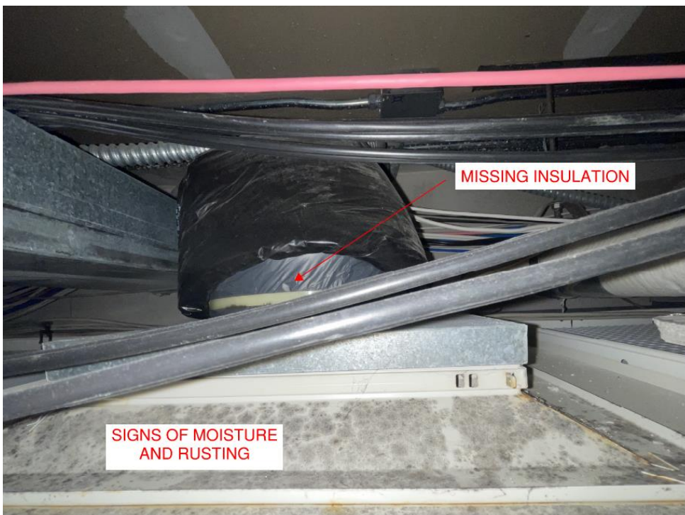
TYPICAL LOCATION IF INSULATION MISSING AT CONNECTION TO DIFFUSER AND MOISTURE ON DIFFUSER CONE.
