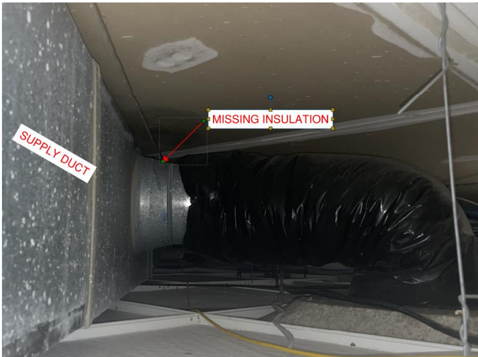
TYPICAL LOCATION OF INSULATION MISSING ON SUPPLY DUCT BRANCH TAKE-OFF TO SUPPLY DIFFUSER.
