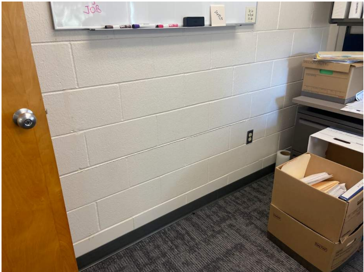
Photo 10: Horizontal CMU crack on office 118 west wall
