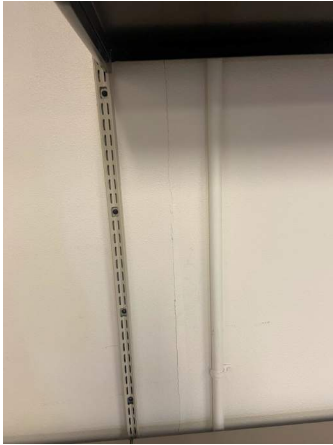
Photo 13: Vertical drywall crack on the south wall of room 117
