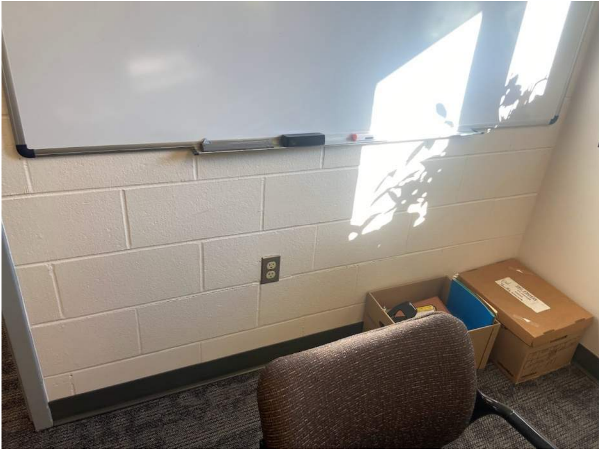
Photo 9: Horizontal CMU crack on office 118 south wall
