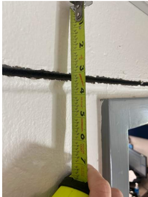
Photo 8: South wall of office 117 and 118 with 3/8" settlement above doors
