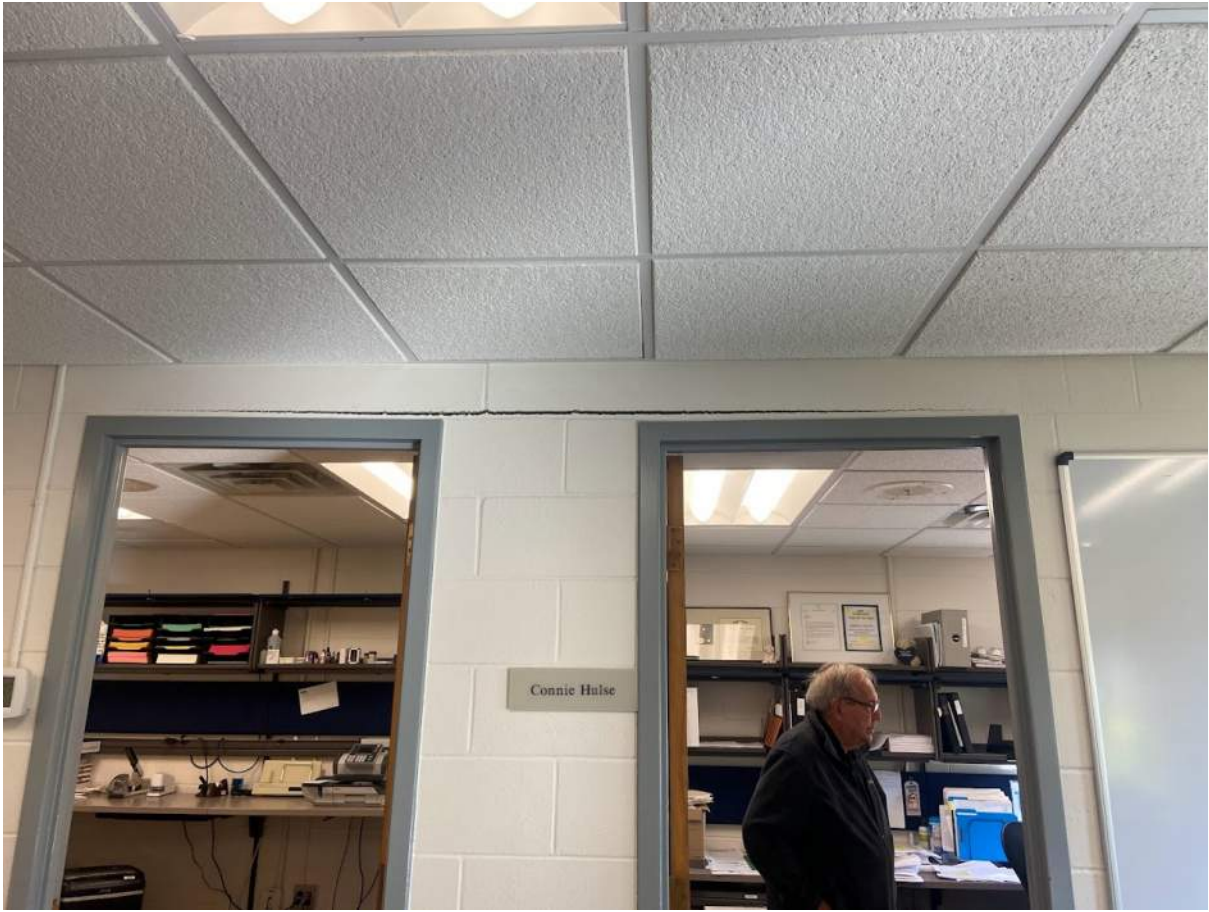
Photo 7: South wall of office 117 and 118 with 3/8" settlement above doors
