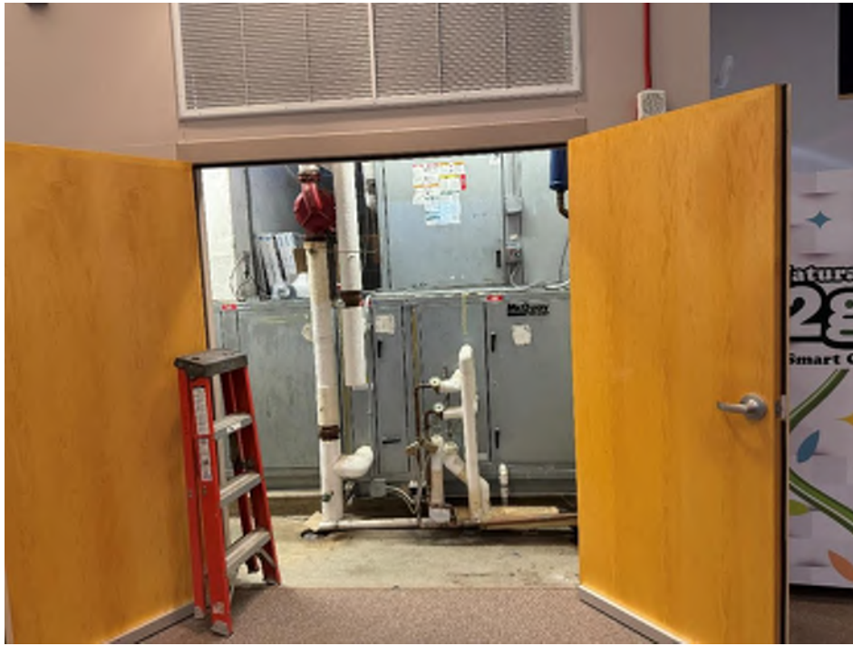
View of the Auditorium HVAC closet.
