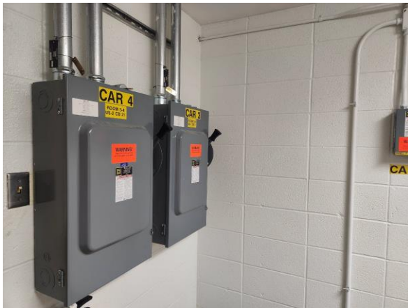
Photo #9 Example of electrical panel in Main Building.
