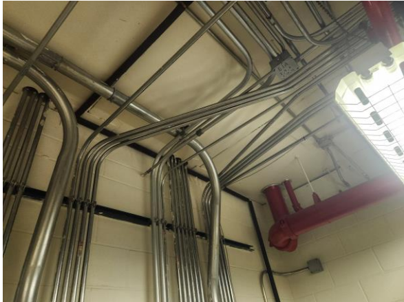
Photo #13 Example of utility runs in Building T.
