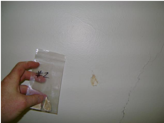
Photo #3 Lead-based paint (white) – CMHI gym plaster ceiling. (6.4%)
