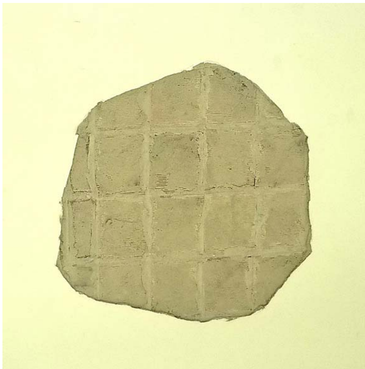
GYM CEILING PLASTER DAMAGE
