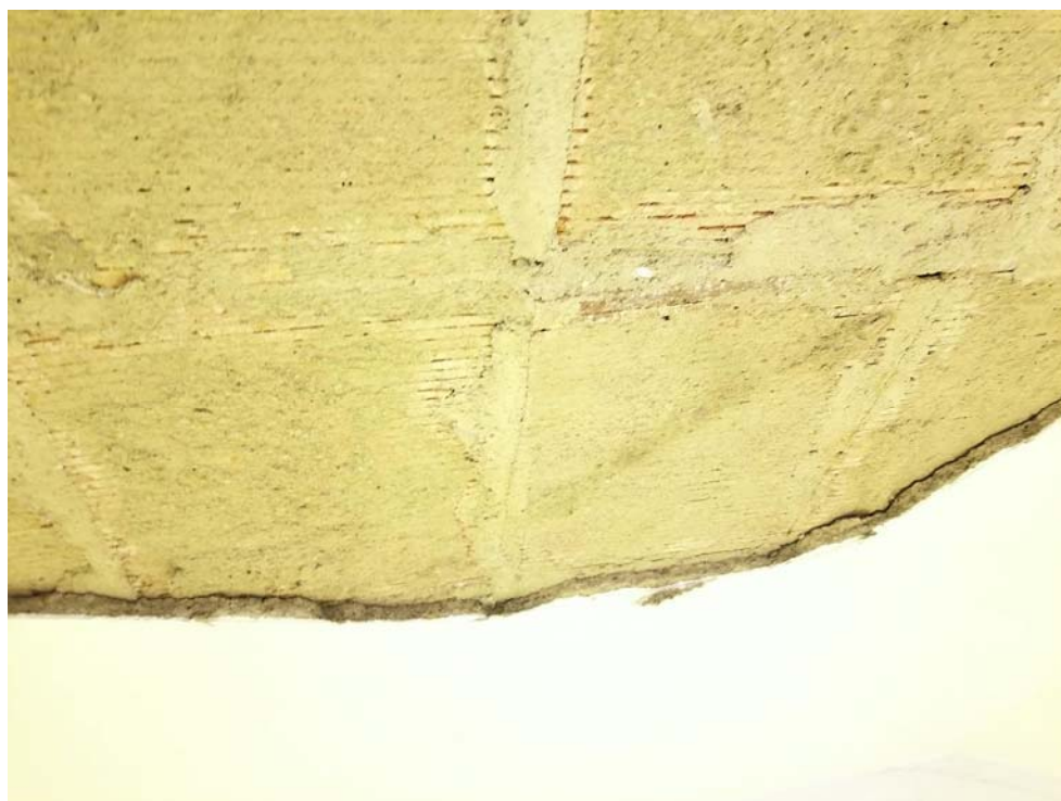
CEILING PLASTER DAMAGE WITH STRUCTURAL CLAY TILE
