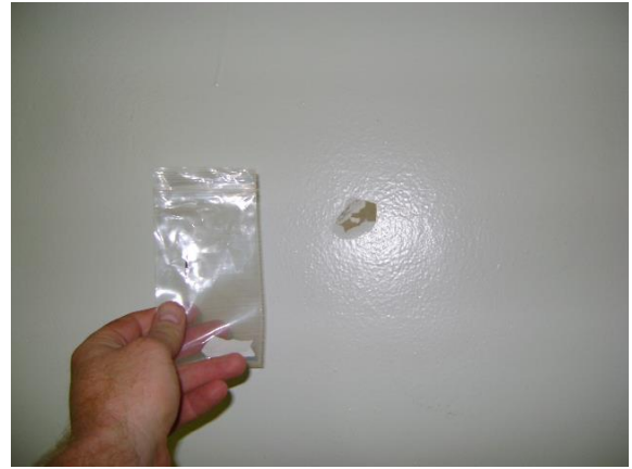
Photo #2 Lead-based paint (white) – CMHI gym plaster west wall. (4.9%)
