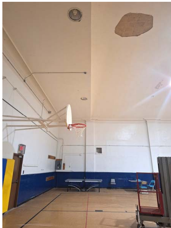
SOUTH END OF GYM WITH CEILING PLASTER DAMAGE
